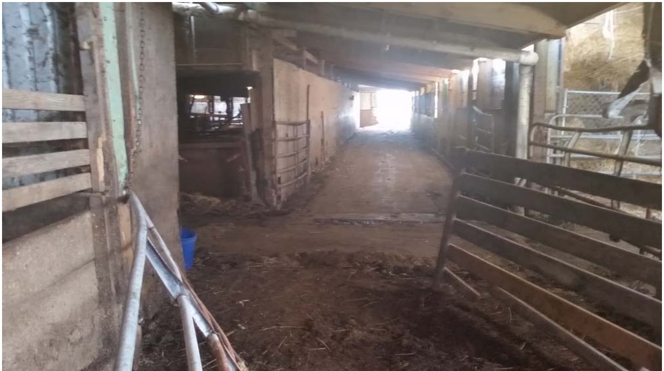
PHOTO 12: West breezeway in loafing shed. Underground liquid manure tanks are located beneath floor.
