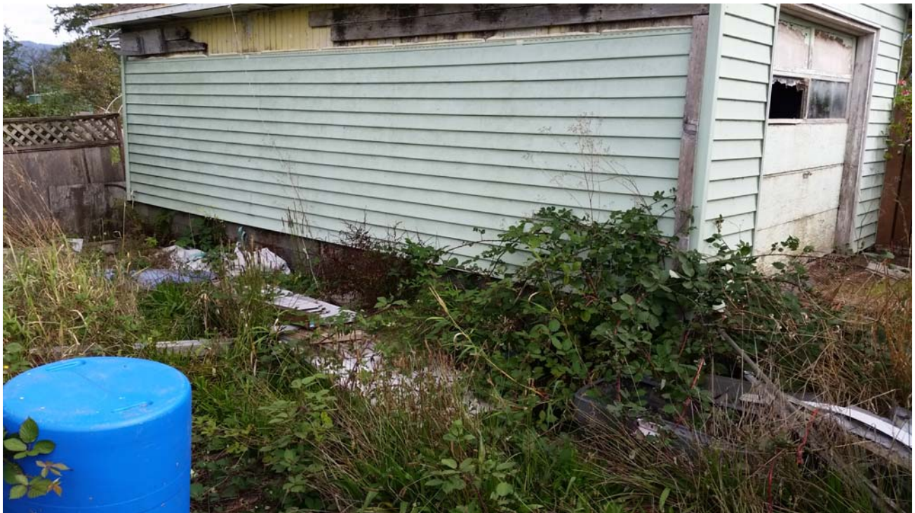
PHOTO 25: West side of garage where above-ground gasoline storage tank was reportedly located.
