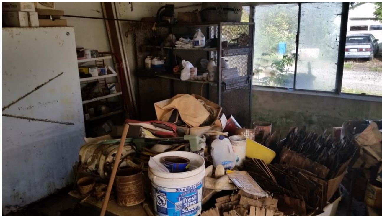
PHOTO 10: Miscellaneous items stored in former milk room. Silt and debris on floor are from most recent flooding event.
