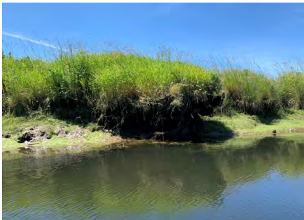
Image 15: Sloughing undercut bank at edge of roadway
