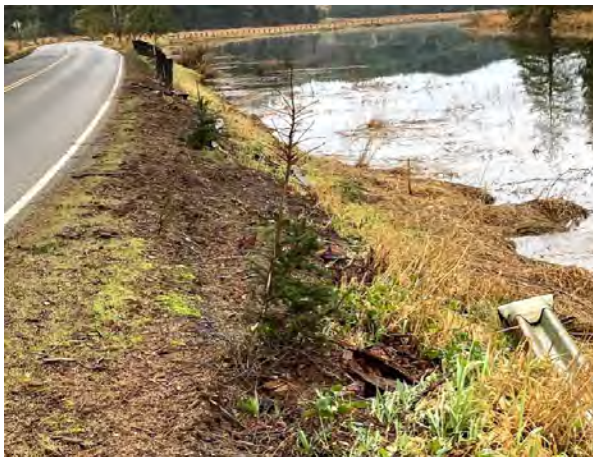
Image 13: Missing guard rail due to recent traffic accident
