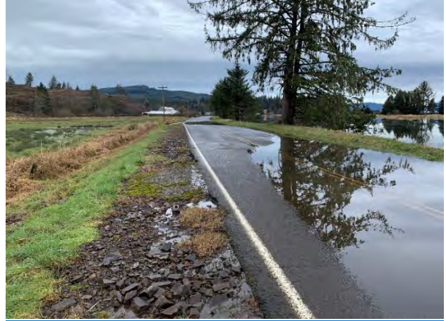
Image 12: Severe cross slope on Burton-Fraser Road due to non-uniform sinking of roadway
