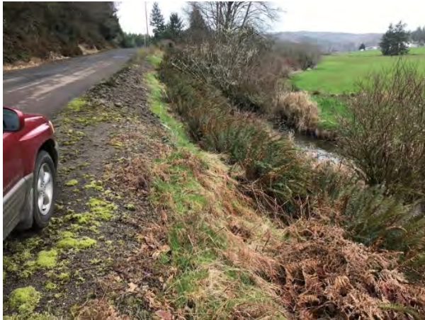
Image 19: Slumping section on eastern 1.5 miles of Eckloff Road
