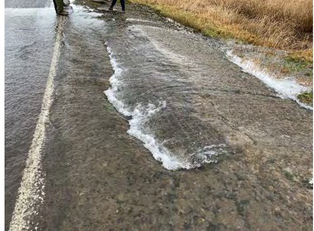
Image 10: CDF Apron with overflowing water during moderate high tide event along TRW, January 27, 2021
