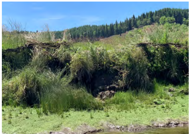
Image 16: Sloughing undercut bank at edge of roadway
