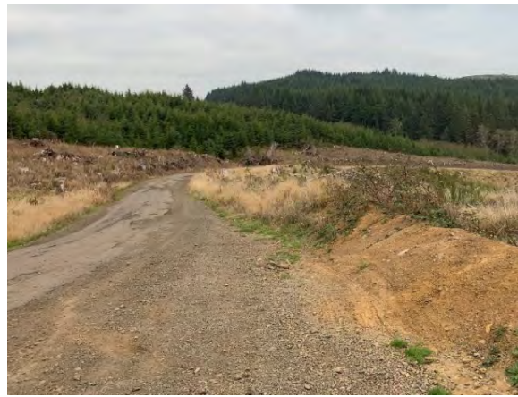
Image 24: Eastern ¾ miles of Eckloff Road rough forest road with steep grade, sharp curves
