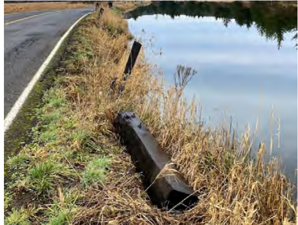
Image 14: Loss of cable barrier posts due to rotting and bank erosion
