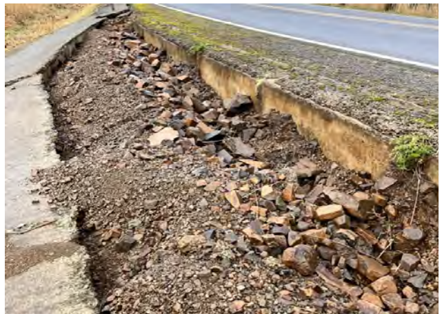
Image 8: Damaged CDF scour protection apron creating abrupt edge hazard
