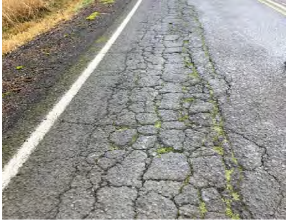
Image 11: Crocodile cracking in pavement, a condition prevalent along Burton-Fraser Road due to underlying settlement
