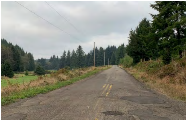
Image 21: West of Beaver Creek Bridge road condition degrades
